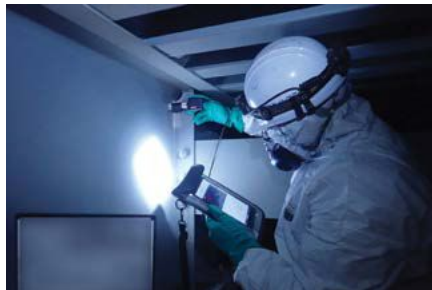
The Coverage Checker Ultraviolet Light Version by TOYO SEIKO at a steel bridge repair work site.
